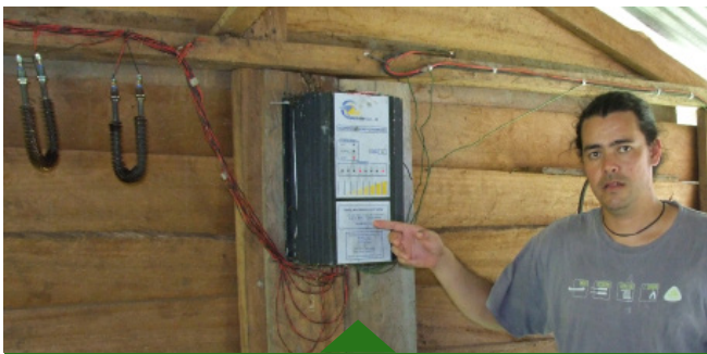
Generator sets and wiring system for electricity
