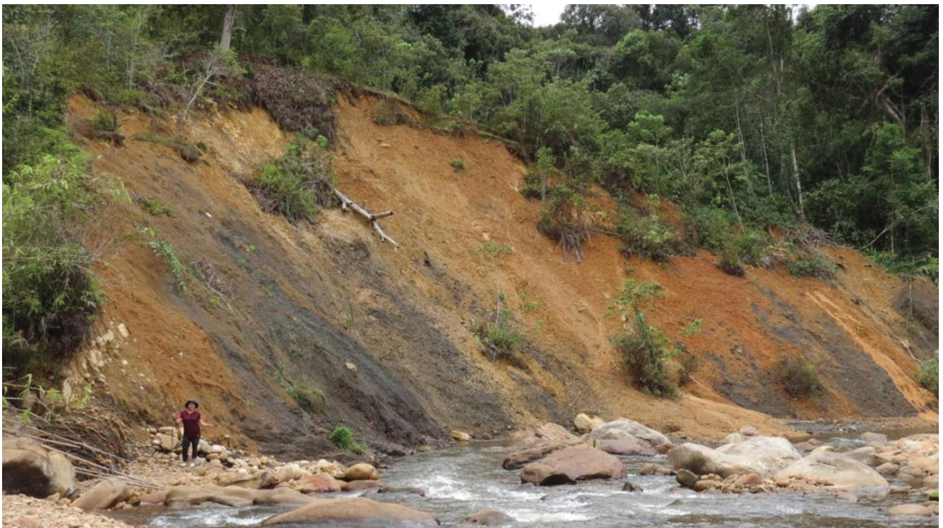
Close up pix of the erosion and landslide at the slope next to the river.
